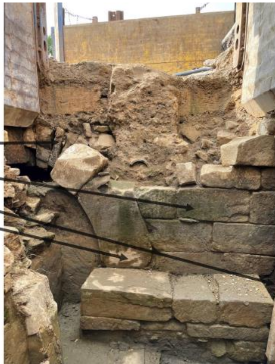
Fig. 4 Roudnice nad Labem, Gothic bridge. Drawing of reconstruction of the structure of the pillar and the semicircular vault. 1) basalt boulder pavement 2) facing ashlars 3) bond-stone 4) slot for lifting mechanism 5) hole called 'vkl' (tame) or 'wolf's mouth' for attaching the metal lifting mechanism called 'vkl' or 'wolf' 6) dovetails on the floor area of arch stones for distribution of mortar 7) supposed sheet-pile wall 8) sheet pile 9) raising of the horizontal grid 10) wooden floor 11) columns attached to the outer side of the horizontal grid 12) base of ballast 13) hypothetical limits of the reservoir 14) axial girder of the wooden horizontal grid 15) transverse anchorage of planks 16) offset of the pillar 17) bossed ashlar of the pillar 18) ledge of the mouth of the pillar 19) roof of the mouth of the pillar 20) water level 21) the top arch stone of a segment of the semicircular vault 22) handrail of the bridge. Drawing: M. Čihla
